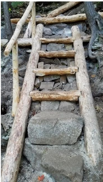
Timber-Rock Hybrid Stairs Constructed on the Bryce Path at Echo Lake SP
