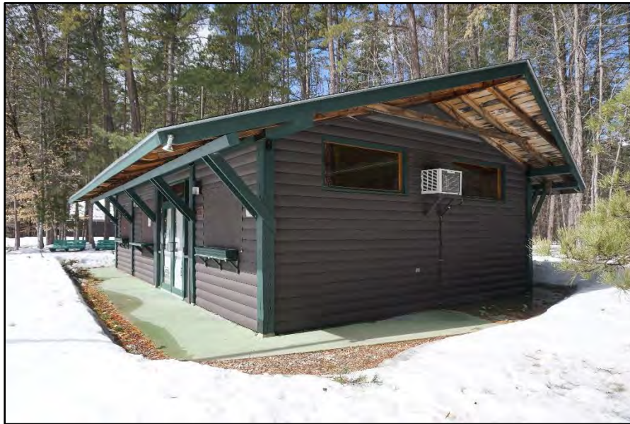
White Lake State Park Office, as seen today. End closest to camera was originally open.
